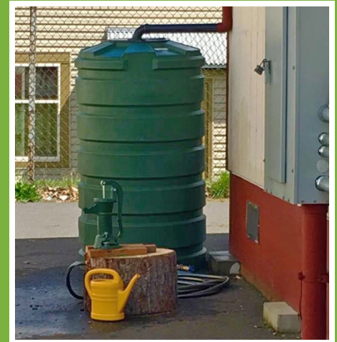
To address water use, a cistern and handpump were installed to collect water off the roof of a portable classroom.
